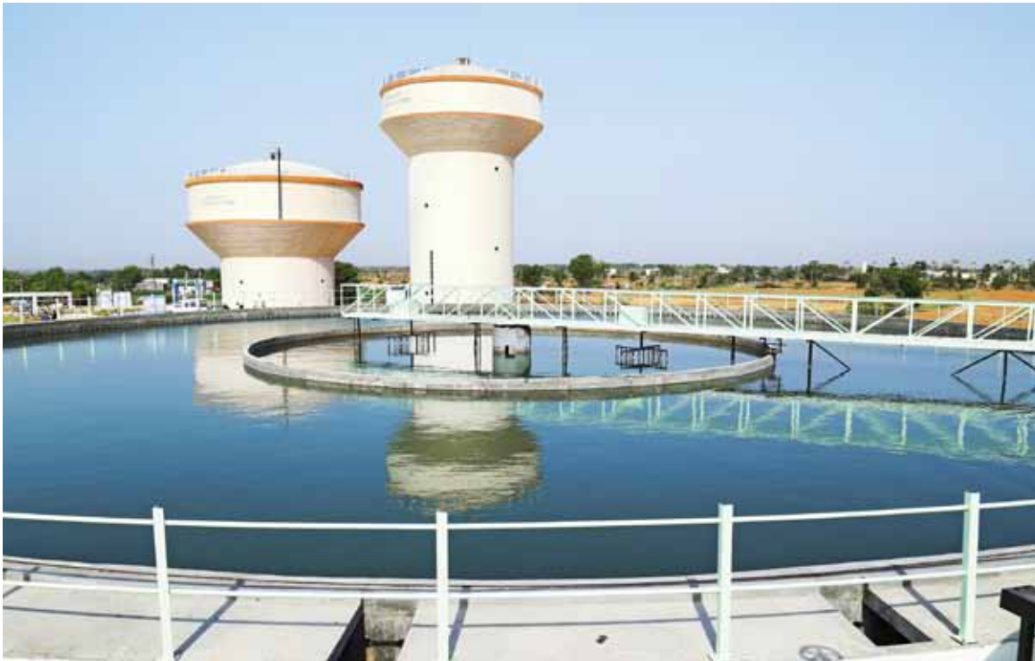
Left: A water treatment plant and clear water reservoir at Dantiwada, Gujarat
